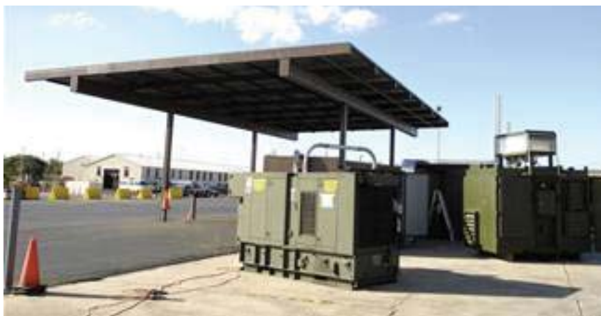
This hydrogen fueling station, partially powered by PV at Hickam Air Force Base, exemplifies DOD's interest in renewable fuels
