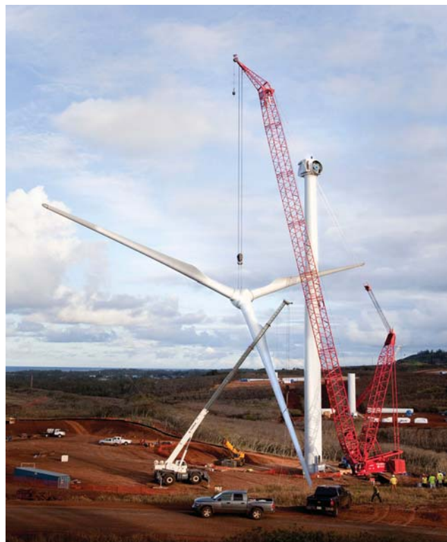
The Kahuku wind farm consists of twelve 2.5-MW Clipper Liberty wind turbines and a 10-MWh Xtreme Power battery storage system.
